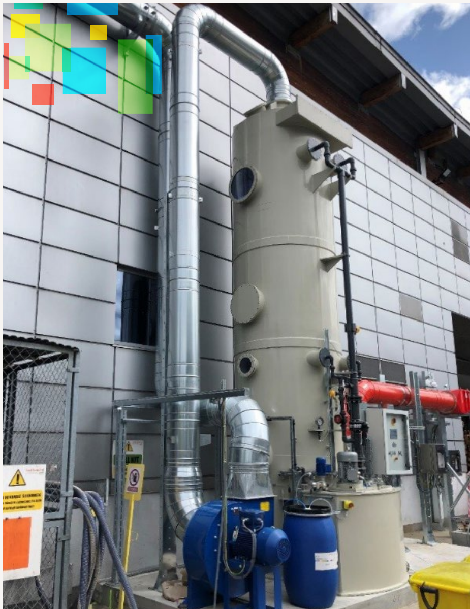
A gas scrubber investment at Sun Chemical Poland improved air quality and production capacity.
