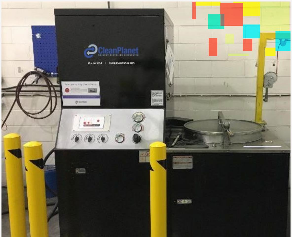
The installation of solvent recycling equipment has played an important role in reducing waste at Sun Chemical.
